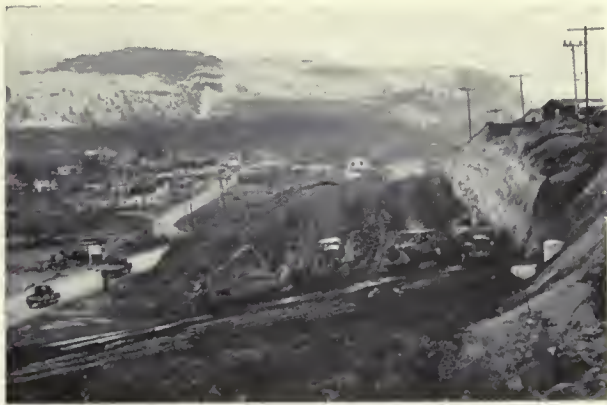
ALL ROADS LEAD TO GRAND COULEE —and the Bureau is building a four-lane highway between Grand Coulee and the top of Grand Coulee Dam. The 1.3-mile strip will use much of the existing road bed. Contractor for the paving job is Goodfellow Bros., Inc., Wenatchee, Wash.
